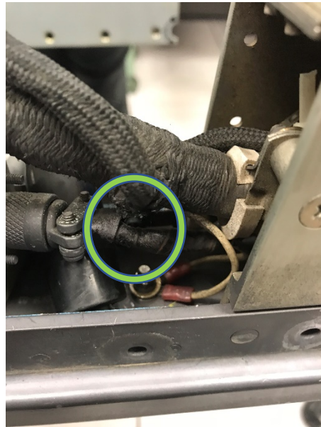
A-10 LAU – Intermittence detected in cannon plug wire connection
